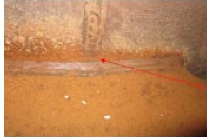
Welding seam is not sufficient.
