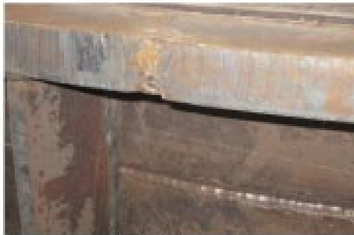
Breach shall be repaired.
